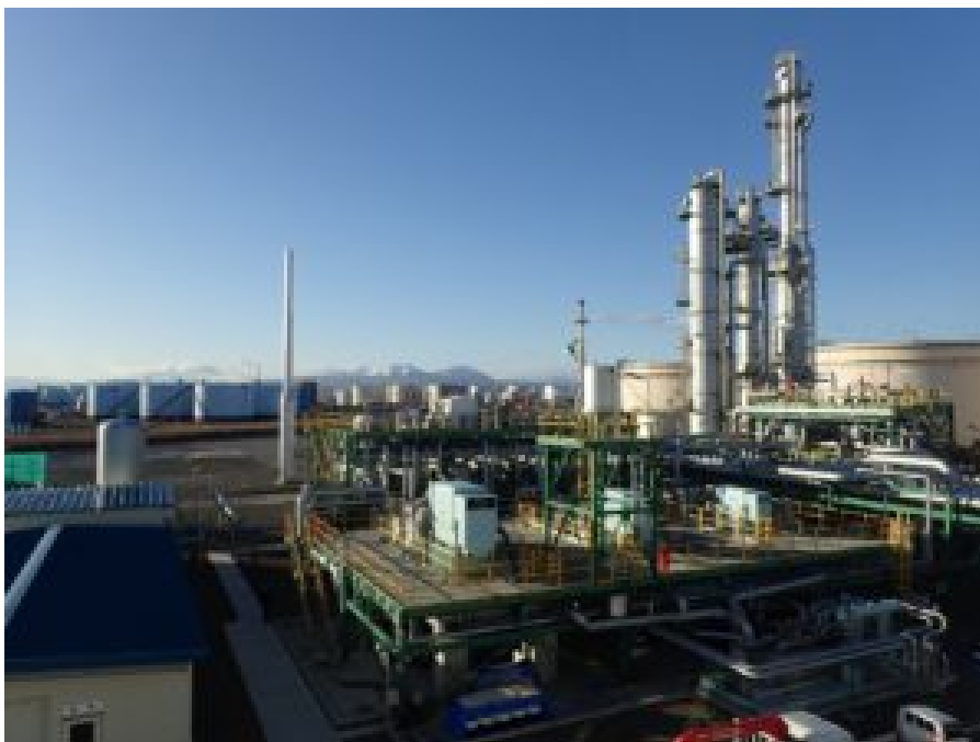
Figure 5: the Tomakomai CCS Demonstration Project Capture and Injection Site
